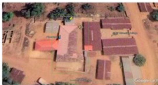
The pre-school area looks to be secured and roof intact, as far as can be seen from the air. Cannot see any tree that could now damage the roof.
